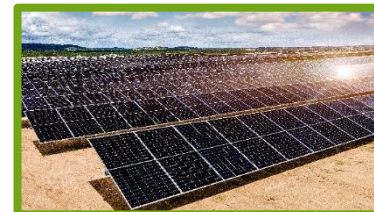
PHOTO: Luzia Solar Complex
