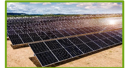
PHOTO: Luzia Solar Complex
